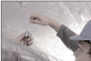
Round Air Ducts
