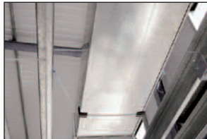
Square Air Ducts
