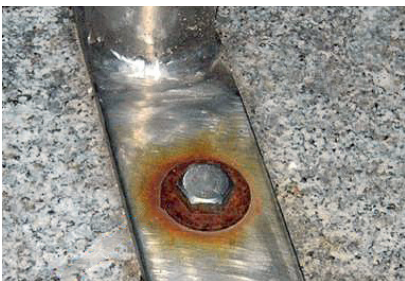
Fig. 12: This is a typical case of contact corrosion. Zinc-plated carbon steel (washer) and stainless steel (screw and part) were used together. The surface area of the more noble metal – the stainless steel – is larger, causing heavy corrosion of the washer.
