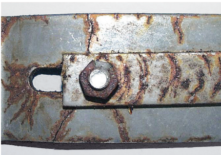
Fig. 8: SCC of a bracket made of the material 1.4301 (A2, 304) after approx. 4 years of use in an indoor swimming pool.
